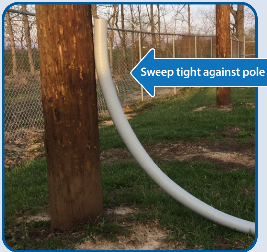
Any radius elbows used shall be 3 feet, 90 degree 2 inch gray PVC sweeps. These sweeps shall be installed flush to OEC pole or stake placed by an OEC Service Planner.
