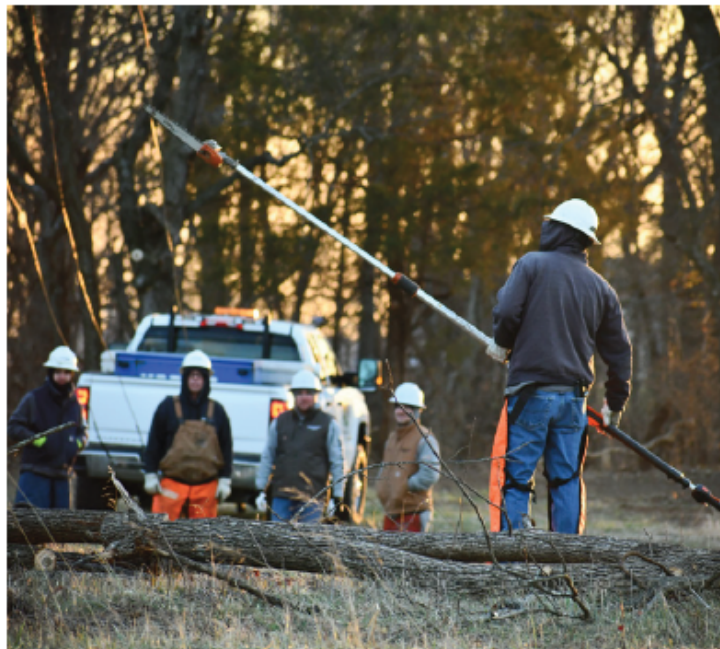
Owen Electric crews participate in a chainsaw operation and line clearing workshop. Linework takes a variety of specialized skills, including the safe removal of trees and limbs from energized lines. Photo: Whitney Duvall
